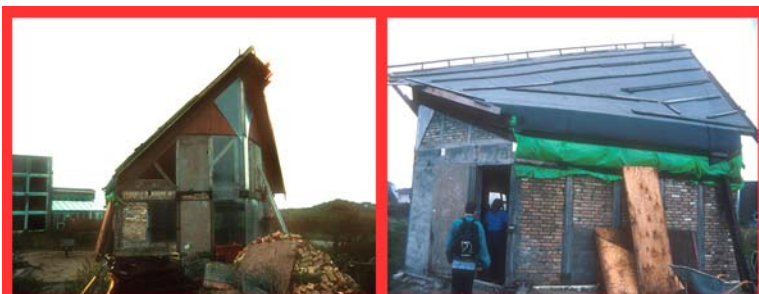
During construction, housing made from scrap materials does not look attractive, however the ambience when completed can be engaging.
